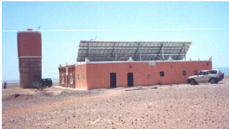
Iferd village (80 electricity meters). The PV central offers electricity (15 hours/day) for individual dwellings and community services (public illumination, school, mosque, etc.). A previously installed PV system provides water pumping.
