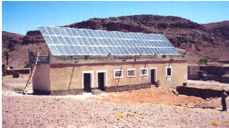
Idboukhtir village (32 electricity meters). The PV central offers electricity (15 hours/day) for individual dwellings, community services (public illumination, school, mosque, etc.) and water pumping.
